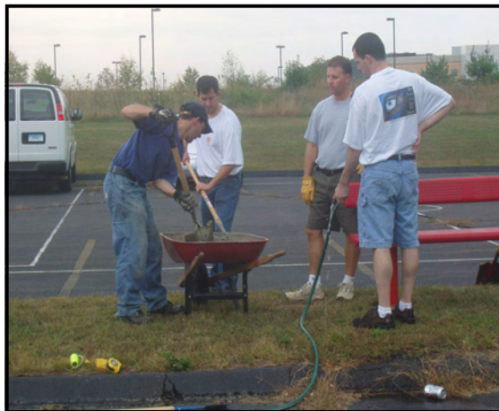
Walker Systems Support employees install a sports bench at the Retreat House
